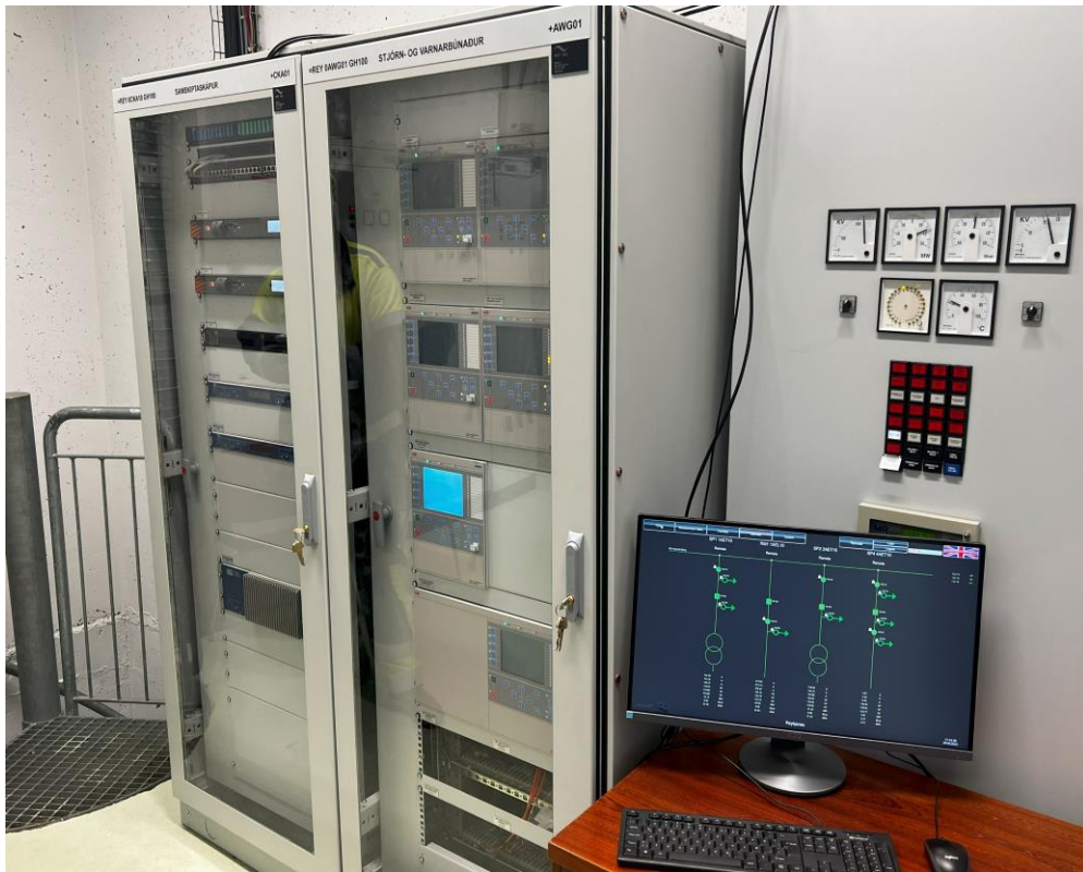
Retrofit geothermal power plant
