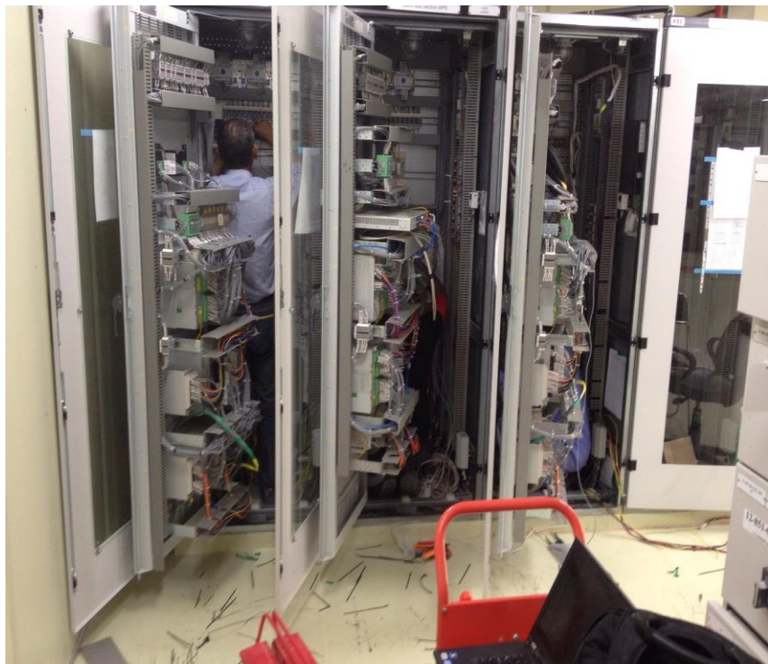
Conventional 132kV Control & Protection incl. Metering for 3 Bays
