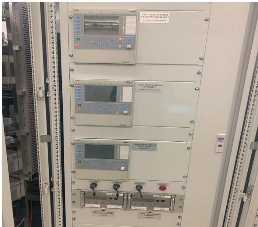
Frontview 132kV Control & Protection incl. Metering for 3 Bays
