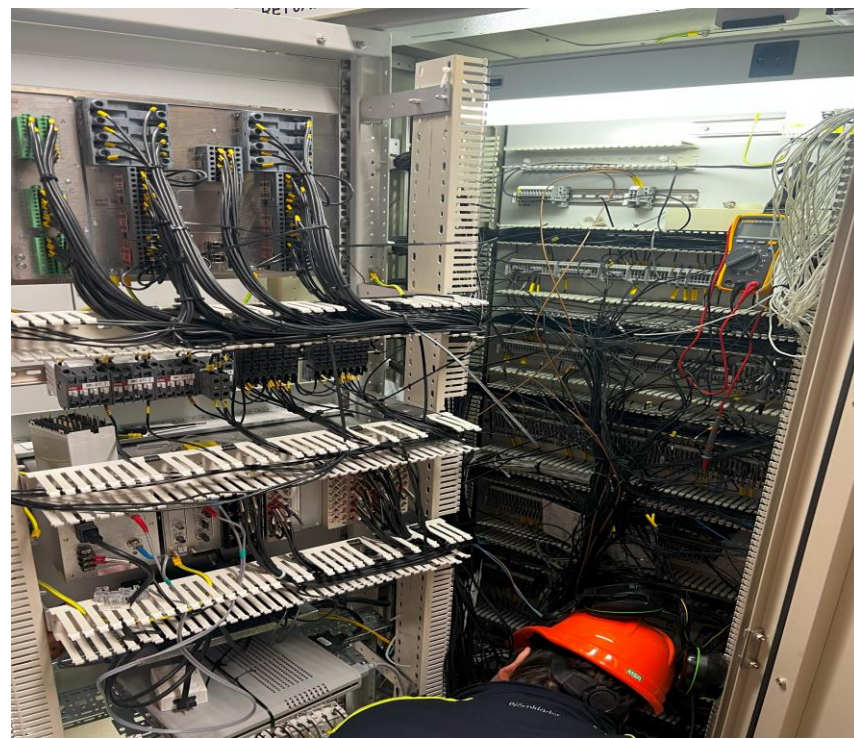
Conventional Control & Protection Cubicle
