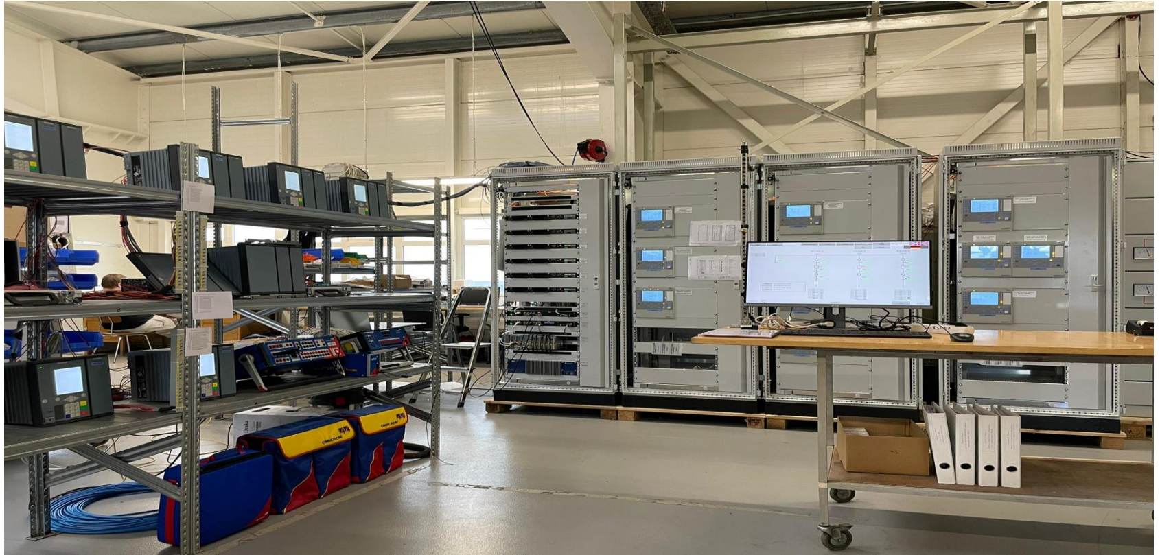
Factory acceptance test in Iceland /Landsnet
