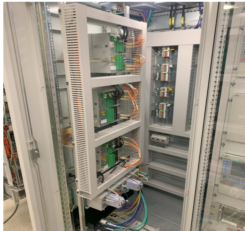
Backview 132kV Control & Protection incl. Metering for 3 Bays
